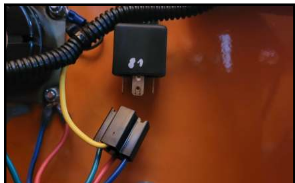
“Unplugged/Disconnected Turntable Ignition Interlock Relay”
